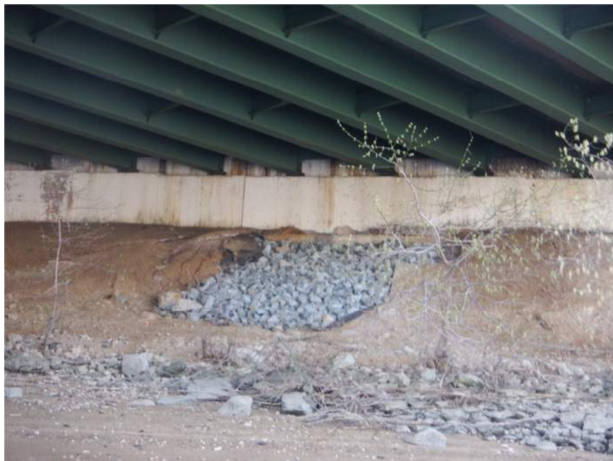
Photograph 6. South Abutment, Looking South. Note: Previous area of erosion has been filled with riprap.
