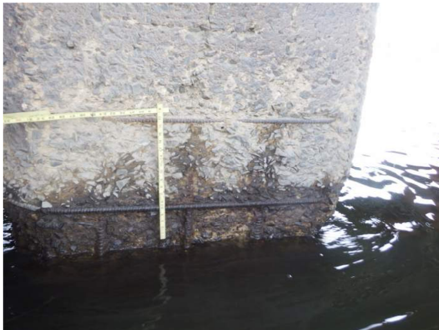
Photograph 4. Pier 5, west face of West Stem, Looking East. Note: 3' H x full-width x up to 4" D scale with exposed steel reinforcement.
