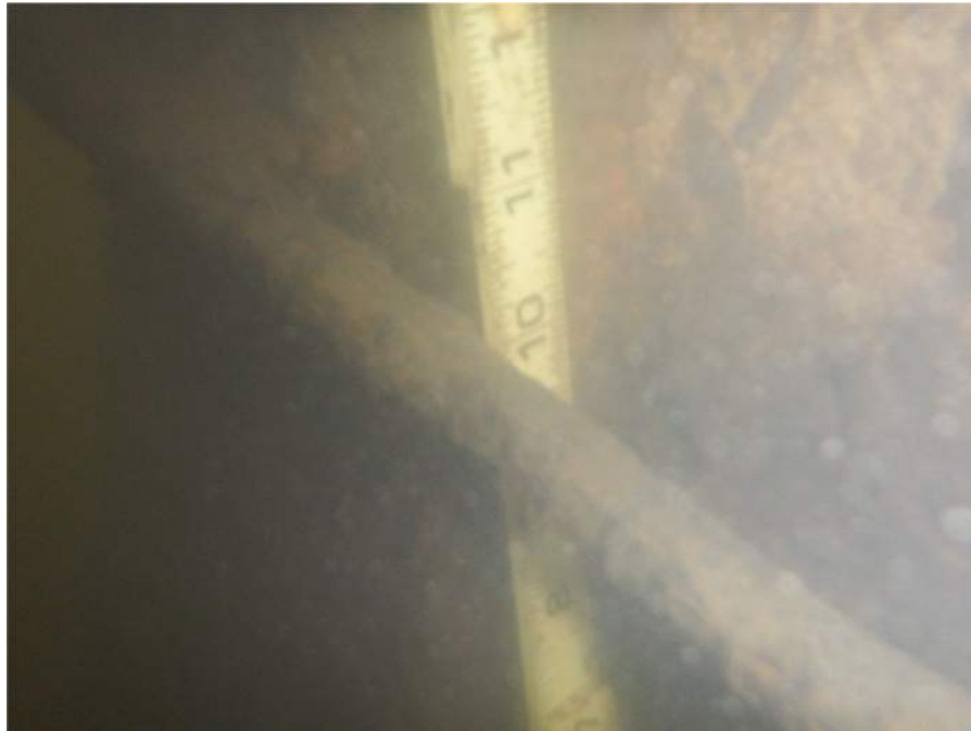
Photograph 5. Pier 5, west face of West Stem, Looking East. Note: Exposed steel reinforcement with section loss.
