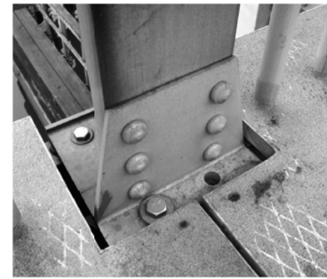
PHOTO 1 NOT TO SCALE MISSING HANDRAIL POST BOLTS; SEE NOTE 1
