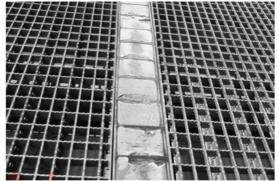
PHOTO 1 NOT TO SCALE VIEW OF EPOXY FILL & INTERMEDIATE PLS. AT DECK LEVEL ABOVE FB1 & FB2; SEE NOTE 1
