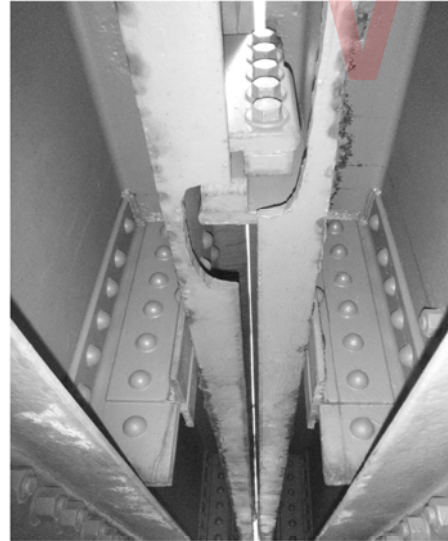
PHOTO 2 NOT TO SCALE VIEW OF THE CENTERING DEVICE SUPPORT CHANNEL & ANGLES FROM BELOW THE DECK AT THE CENTERING DEVICE
