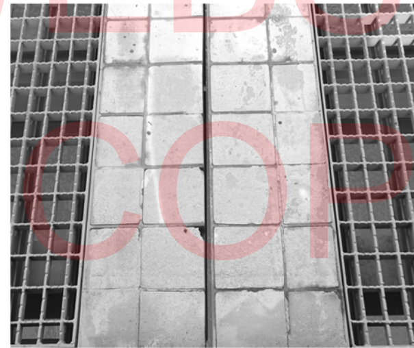
PHOTO 3 NOT TO SCALE VIEW OF THE EPOXY FILL & INTERMEDIATE PLATES AT DECK LEVEL
