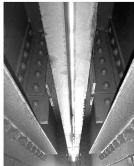
PHOTO 1 NOT TO SCALE VIEW OF THE CENTERING DEVICE SUPPORT CHANNEL & ANGLES FROM BELOW THE DECK
